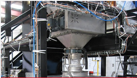
EDF - Turnkey project to ensure compliance of boric acid preparation stations
