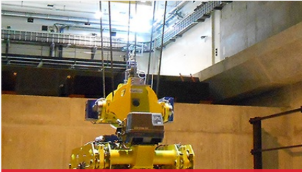
ICEDA facility at EDF Bugey NPP - High- integrity handling equipment
